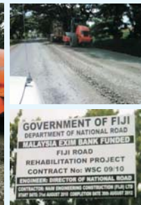
Nadi Back Road Rehabilitation works being carried out by Naim Cedera Ltd -ADFB Funded Project. Standard Concrete Industries supplied 5000m3 of Base Course material for this project.
